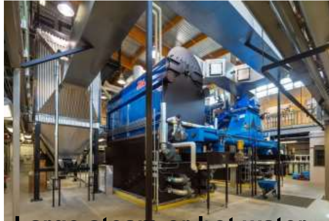
Large steam or hot water boilers
