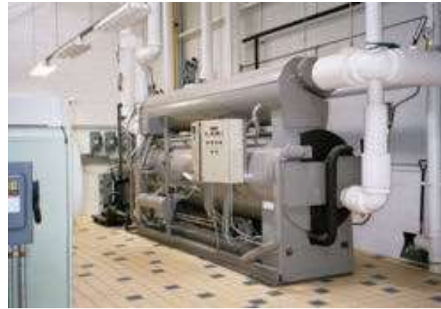
Absorption Chillers for Cooling
